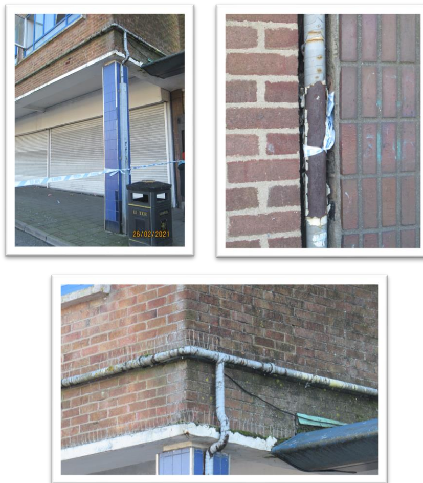
Figure 11a: Countisbury Avenue vertical riser on MOB before replacement
