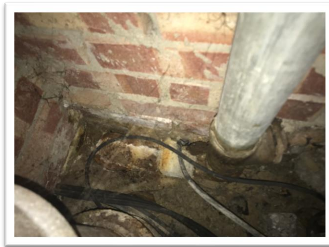
Figure 28: Hatherleigh Court, Swindon MOB Riser 1 before replacement
