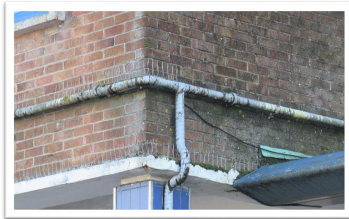
Figure 26: Countisbury Avenue vertical riser on MOB before replacement
