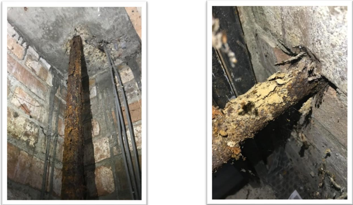
Figure 5: Photographs of corrosion at Northcliffe, Penarth, Wales
