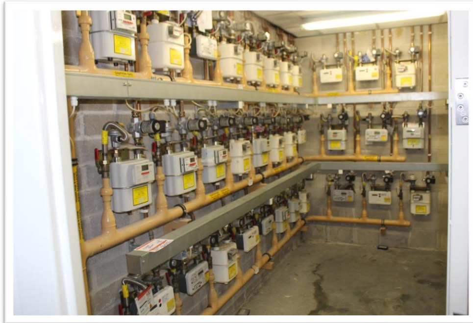
Figure 3: Manifold installation in a dedicated room at ground level
