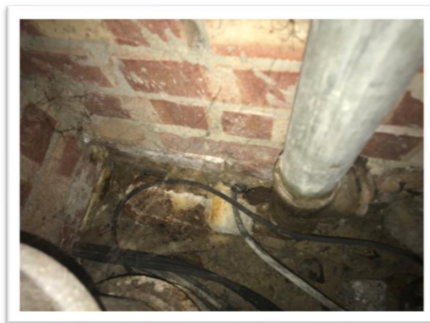
Figure 12: Hatherleigh Court, Swindon MOB Riser 1 before replacement
