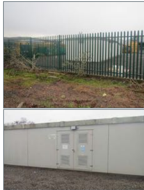
Location C PRS compound (top) and air vents on doors of building (bottom)
